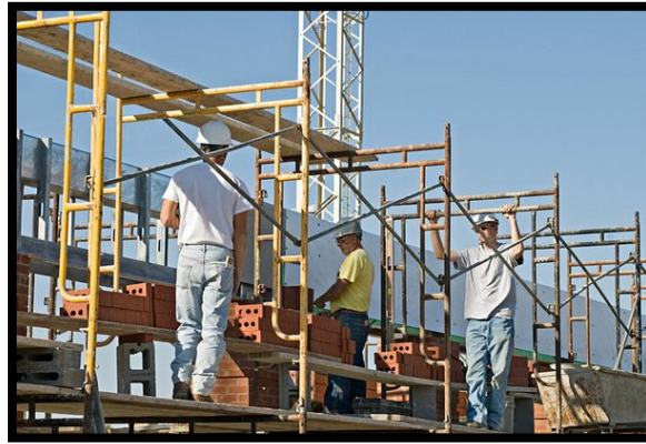
Rajah 4: Sistem Perancah ( Scaffolding )
